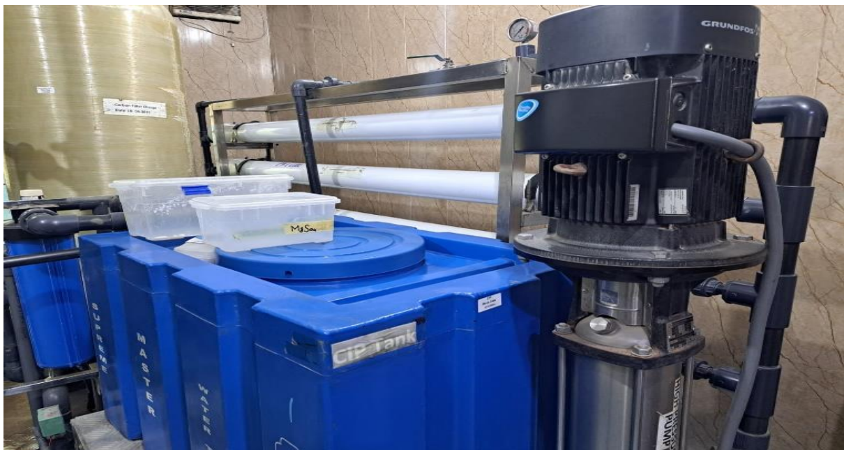
RO Water Plant at UMT
