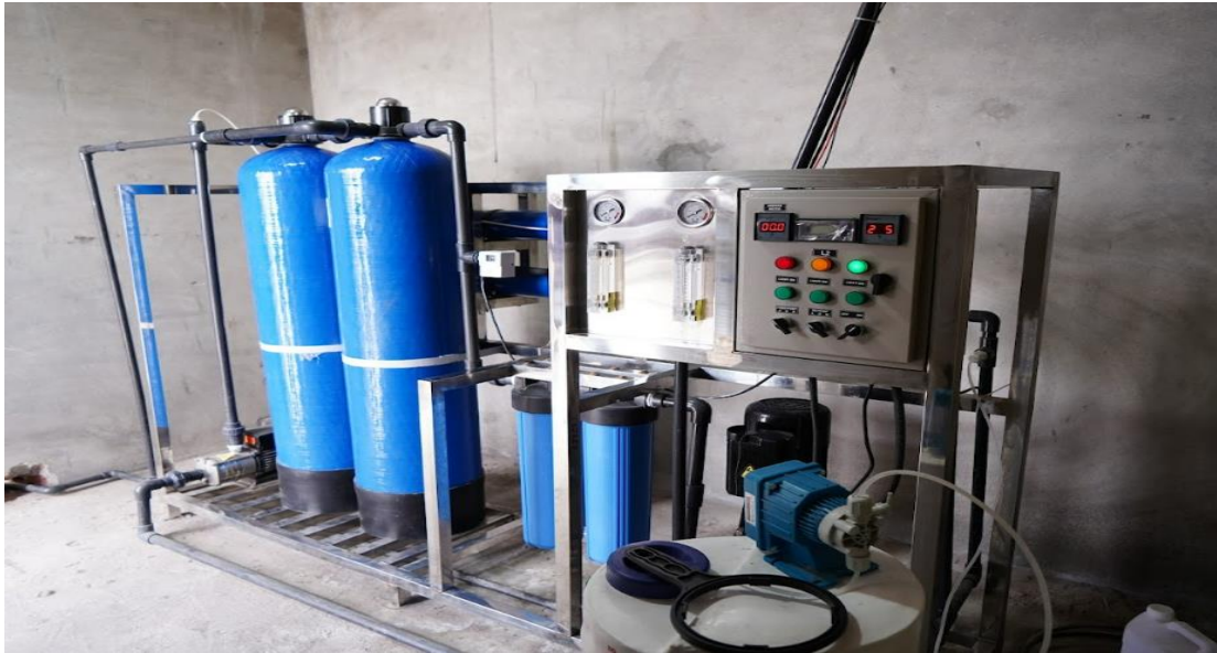
Water purification Plant
